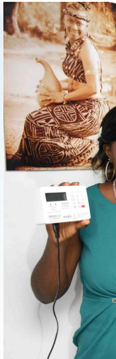
Eneo prepaid solution: more than 7,000 meters installed, as at 31 June 2019
